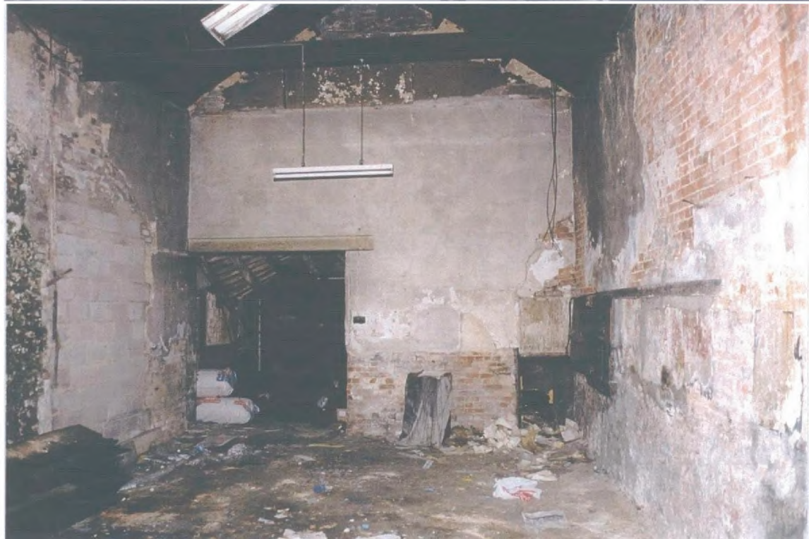
Top: The former façade of Seward's theatre in St George's Place, by then an internal wall, shortly before demolition.
