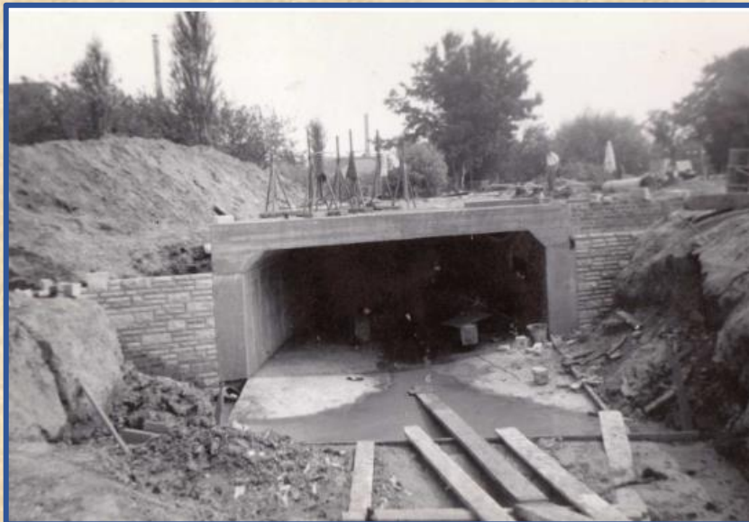
Re-routing of the River Chelt during the construction of Princess Elizabeth Way © Alan Bradley
