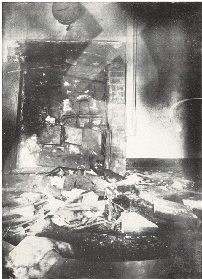
Boiler Explosion at Tewkesbury Rural District Council's Isolation Hospital at Tredington, Jan. 4th, 1908.
