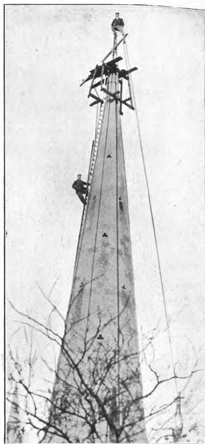
Steeplejacks at work on St. Mark's Church, Cheltenham, 170ft. high, and substituting copper vane for iron.
