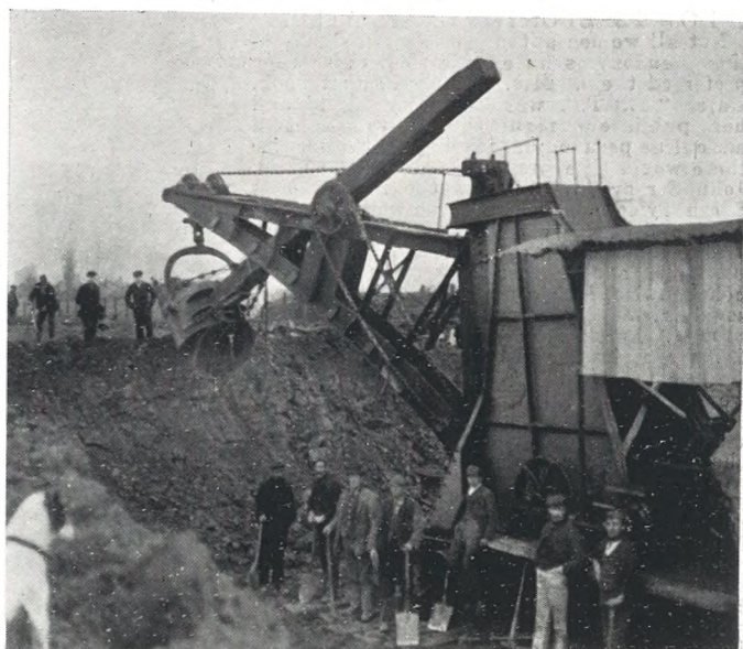
STEAM NAVVY AT WORK AT MARLE HILL COURT FARM, SWINDON LANE, FOR NEW RAILWAY TO HONEYBOURNE.
