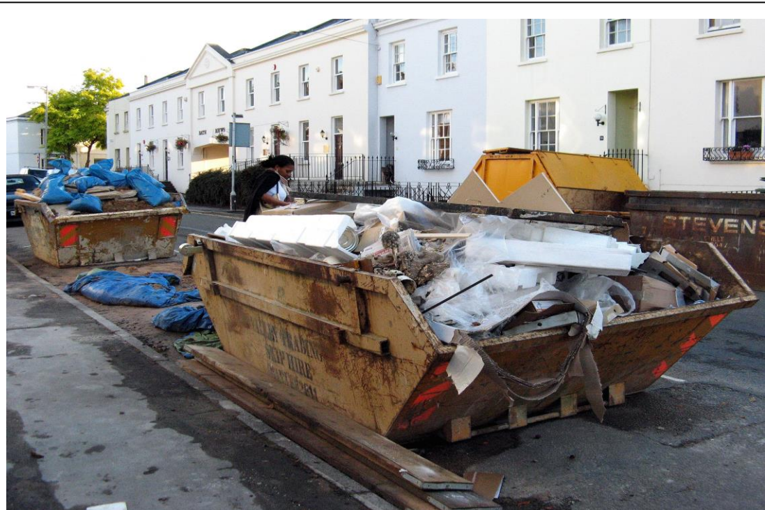
After the floods, Bath Parade, Cheltenham. Repair work was still ongoing in many properties and was to continue for many more weeks, 9 October 2007
